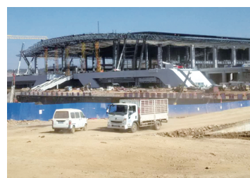
The main building of Kunming HSR South Station is being roofed. Photo by Li Hongbing
