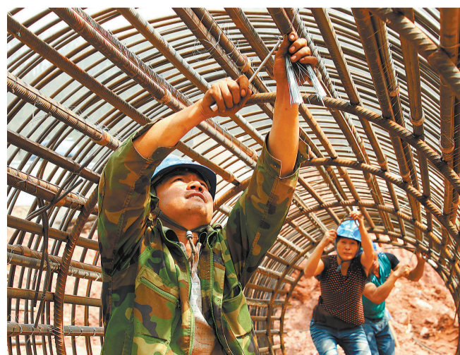
Builders at the construction site of Xiaomo Highway. Photo by Huang Zhechun
