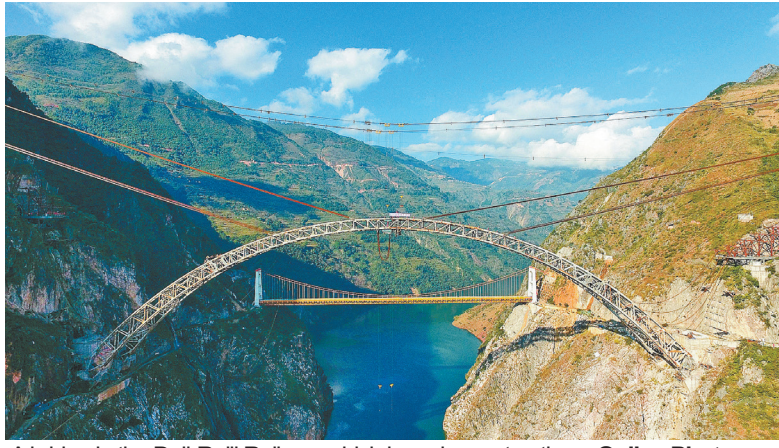
A bridge in the Dali-Ruili Railway which is under construction. Online Photo
