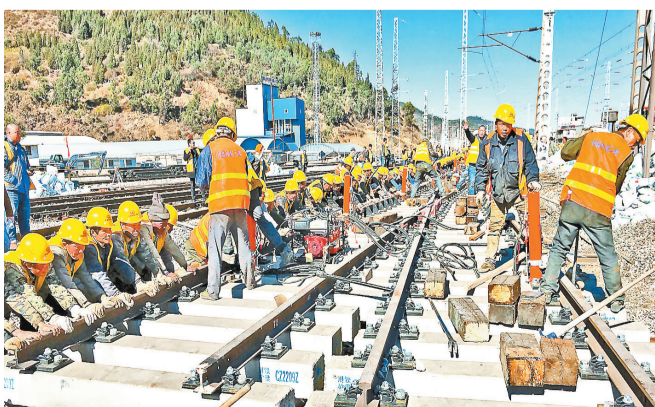
Upgrading works of the Dali Railway Station in west Yunnan are launched on January 7. (Photo by Hu Xiaorong)
