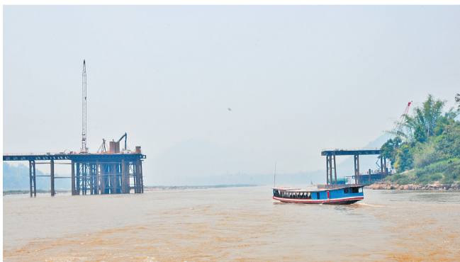
The Luang Prabang railway bridge under construction by China Railway No.8 Engineering Group Co., Ltd. (CREC8) over Mekong River in northern Laos. (Xinhua photo)
