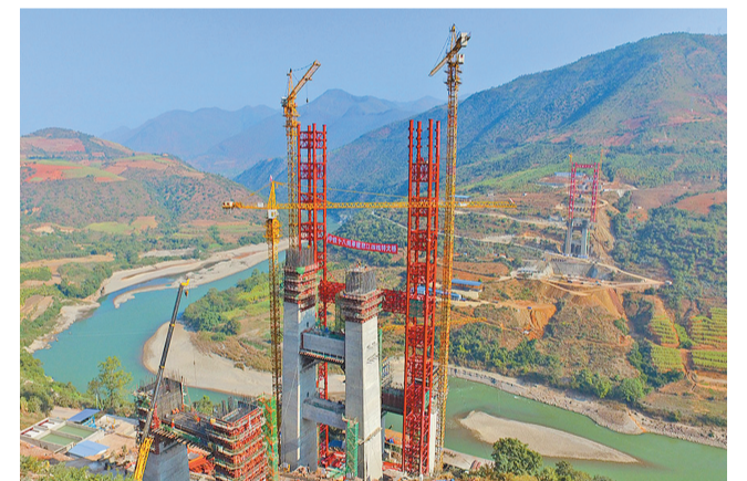
Bridge piers are being built across the Nujiang River in Yunnan, as part of the China-Myanmar railway project. Xinhua photo
