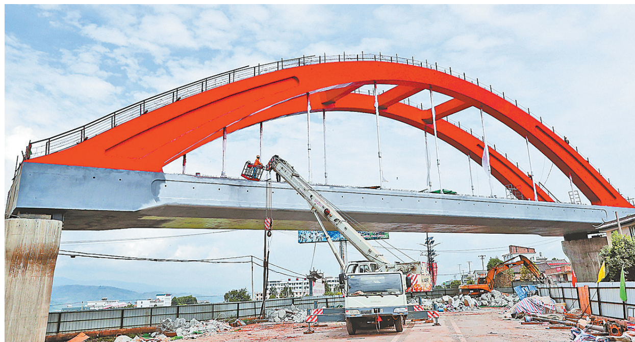
The construction of the tied arch on the Bailong Bridge has recently come to an end in west Yunnan's Weishan County. The bridge is a key project on the 202-km Dali-Lincang railway. With an investment of 15.53 billion yuan, the Dali-Lincang railway is expected to improve the province's connectivity with Myanmar and other neighboring countries. (Photo by Yang Zheng)
