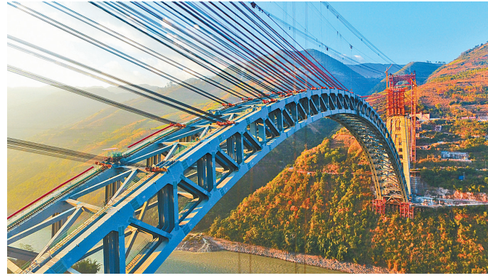
On the morning of December 10 th , 2018, the steel truss arch of the four-track railway bridge on the Nujiang River was completed. The bridge is a key project of the Dali-Ruili Railway in Yunnan Province, and this step marks significant progress in the construction of the China-Myanmar Railway. The steel bridge is the world's longest-spanned railway arch bridge. (Xinhua)
