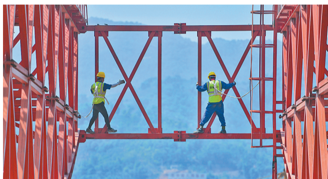
Two workers are fastening bolts on the Munai River Double-track Bridge under construction. (Xinhua)
