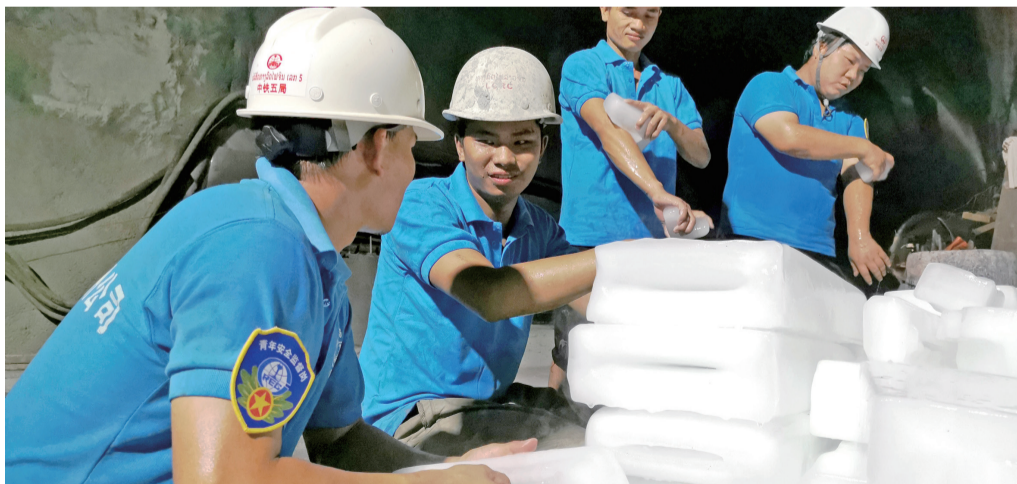
Workers are moving the ice blocks into the Ban Konlouang Tunnel. (Xinhua)
