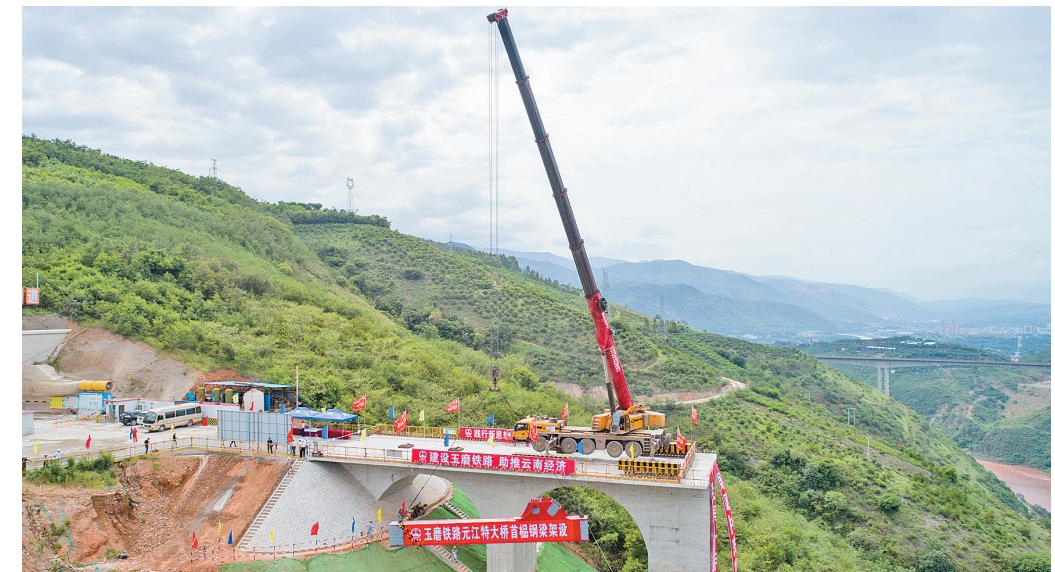
When its construction is completed, the Yuanjiang Railway Bridge will be 832.2 meters long. Photo by Huchao
